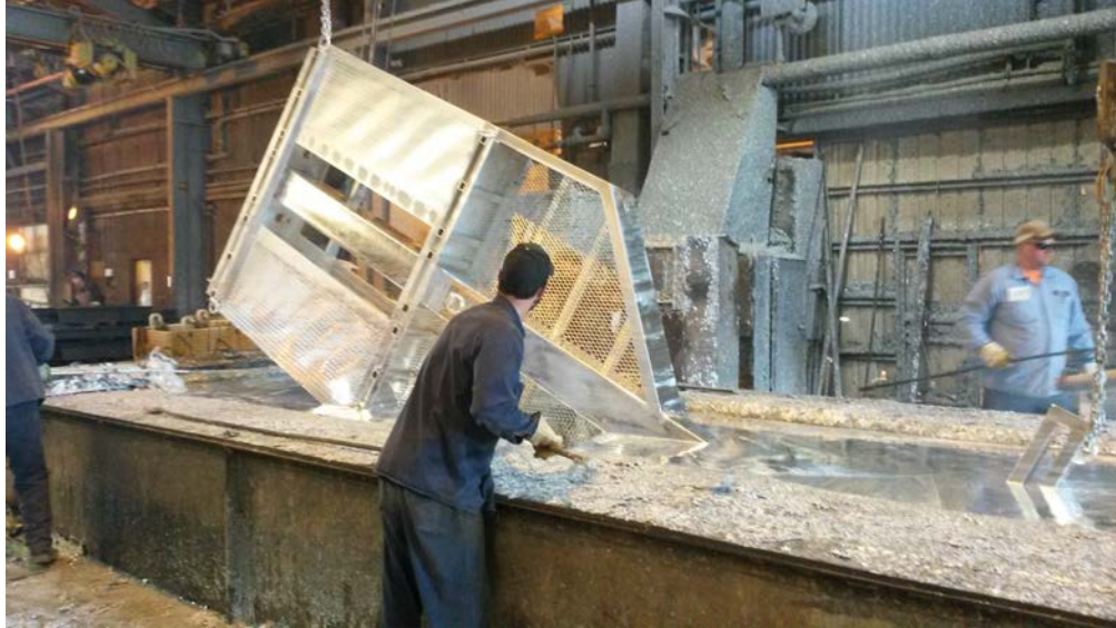
After extensive preparation in acid and caustic vats, the trailer frame is dipped in a kettle full of 800 degree zinc.
